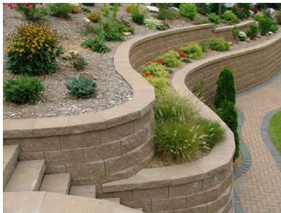
Figure 3-12: Retaining walls shall be benched, or terraced, so that no individual wall exceeds a height of six feet.
